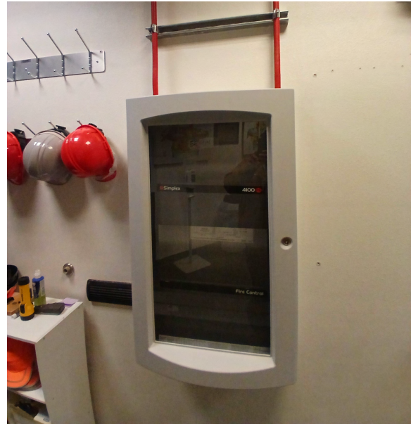
New fire safety control panel installed in the LBT lobby. Photo Credit: T. Castro
