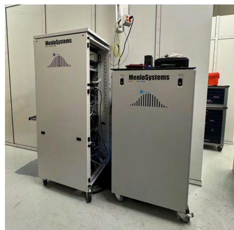
The cabinets housing the new LFC on level 1 at the LBT.
